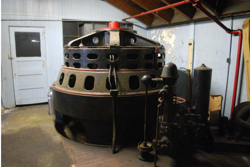
Figure 4. Existing Hunt's Mill Generator and Governor
