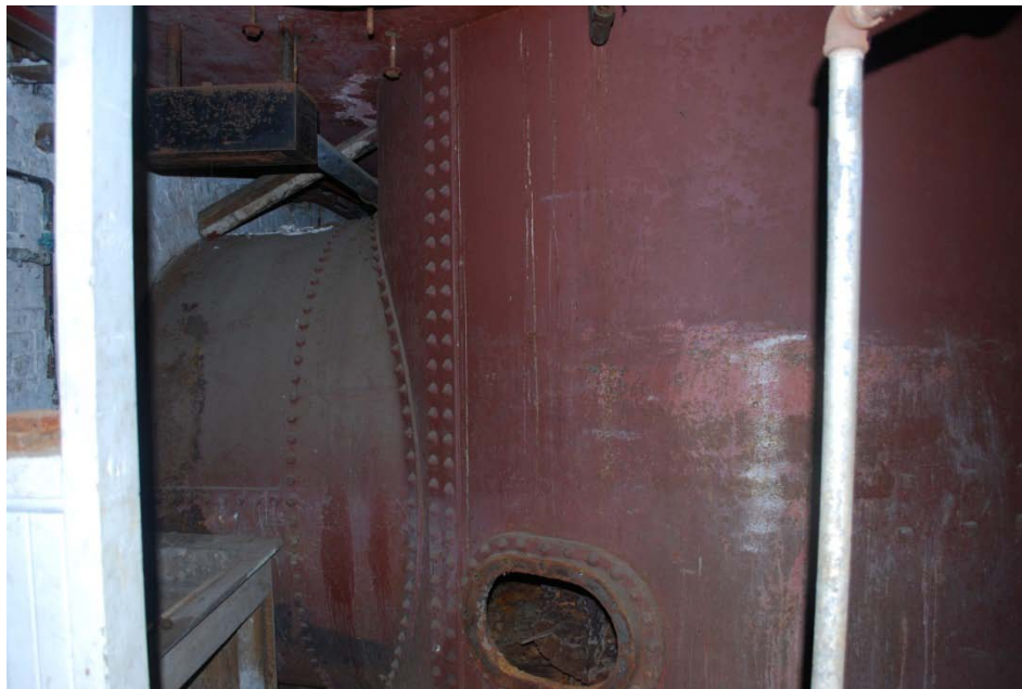
Figure 5. Steel penstock and Vertical Pressure Case
