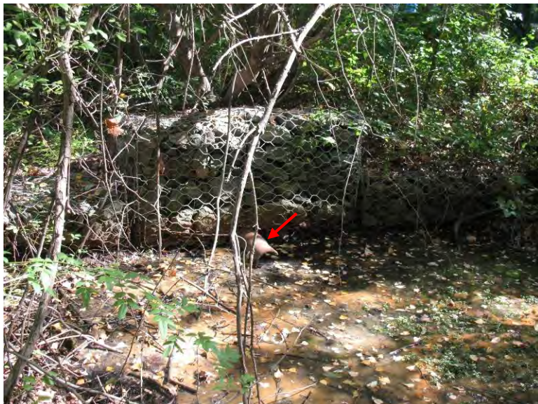
Photo 6. Turner Reservoir Dam. Stone gabion wall with drain pipe outlet (arrow) at toe of left embankment.
