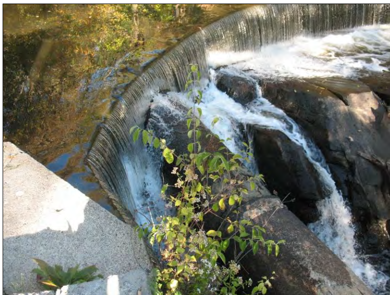
Photo 9. Hunt's Mill Dam. Abandoned power penstock at spillway toe.
