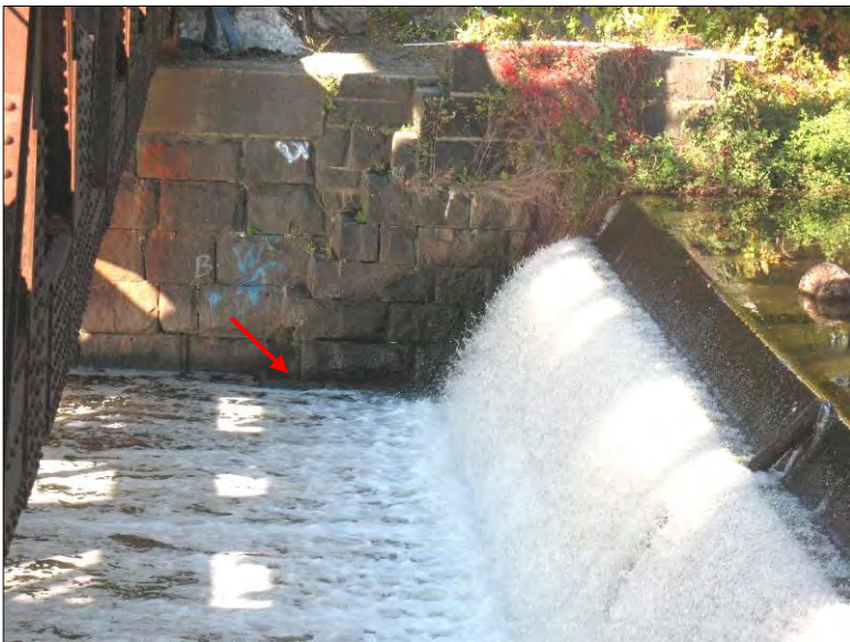
Photo 21. Omega Pond Dam. Right dam abutment from left abutment wall. Note open masonry joints , missing stone step at bottom (arrow) and vegetation.
