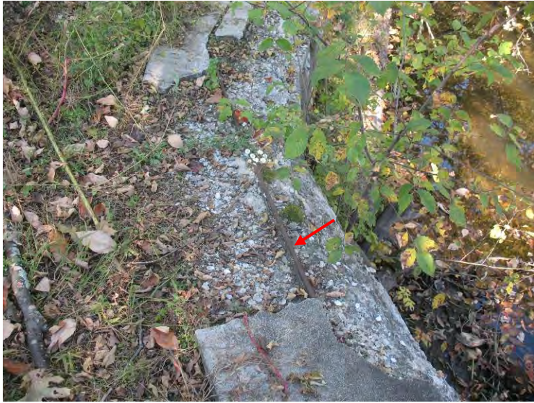
Photo 16. Hunt's Mill Dam. Deteriorated concrete with exposed reinforcement on top of upstream retaining wall (arrow).
