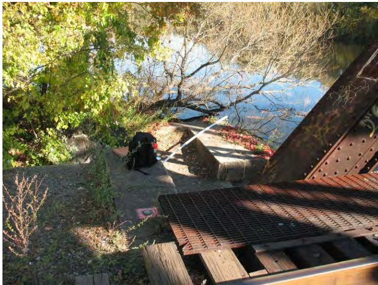
Photo 20. Omega Pond Dam. Top of right dam masonry abutment from railway bridge.
