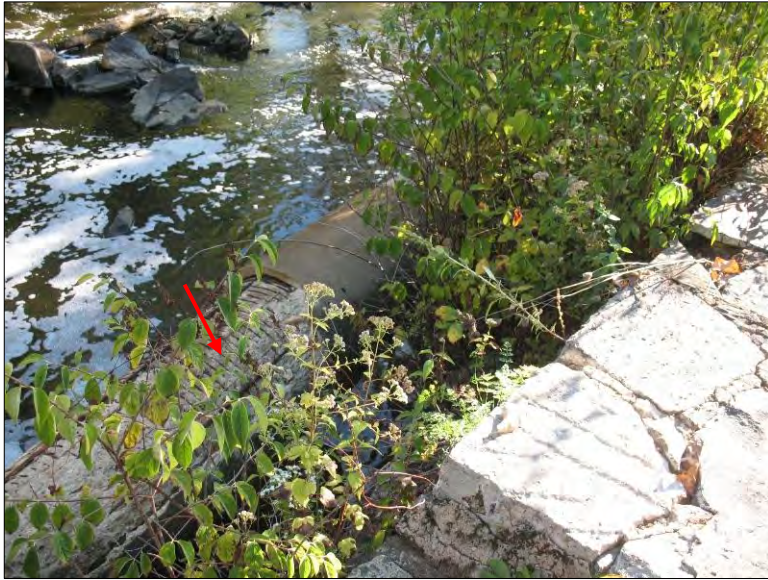
Photo 10. Hunt's Mill Dam. Deteriorated concrete section of abandoned penstock (arrow).
