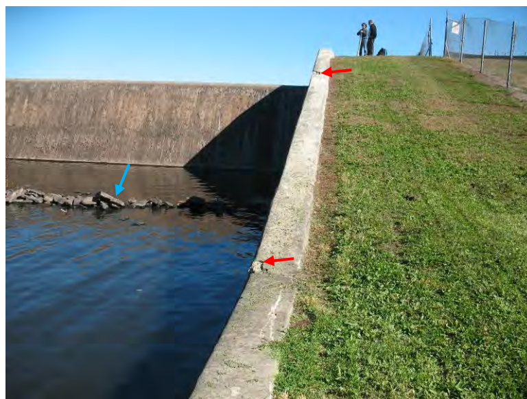
Photo 3. Turner Reservoir Dam. Left retaining wall. Note areas with concrete deterioration (red arrows) and pile of stone in tailwater (blue arrow).
