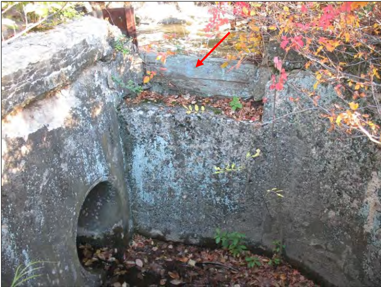
Photo 11. Hunt's Mill Dam. Concrete chamber interior with upstream penstock inlet on bottom and waste weir with wooden planks in riverside wall (arrow). Note concrete wall deterioration.
