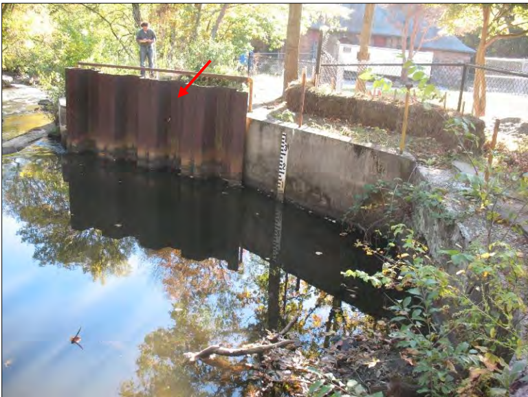
Photo 12. Hunt's Mill Dam. Upstream view of abandoned headrace entrance closure wall (arrow).
