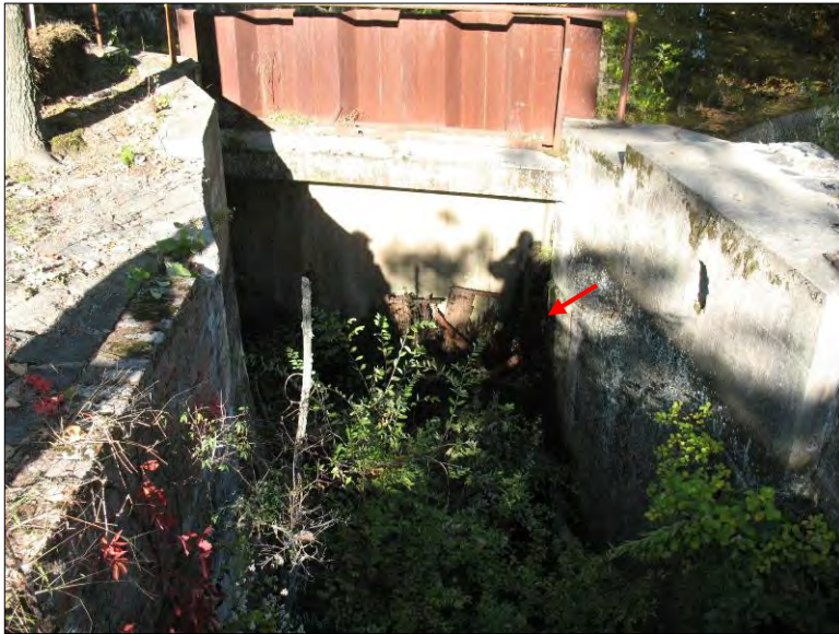
Photo 13. Hunt's Mill Dam. Downstream view of abandoned headrace closure wall leaking at left corner (arrow).
