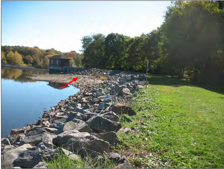
Photo 7. Turner Reservoir Dam. Right dike looking toward gatehouse. Note upstream slope area with missing riprap (arrow).
