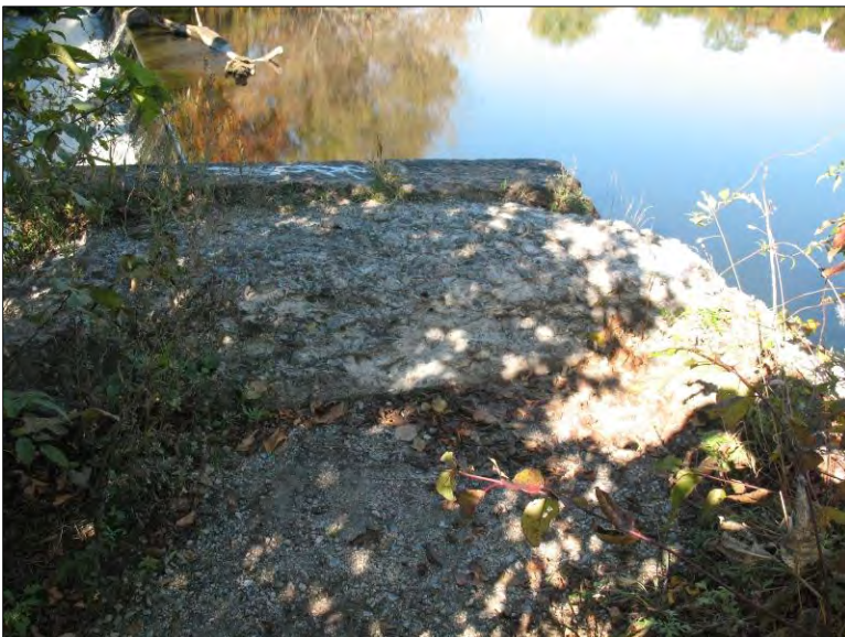
Photo 18. Omega Pond Dam. Deteriorated concrete on top of left masonry abutment.
