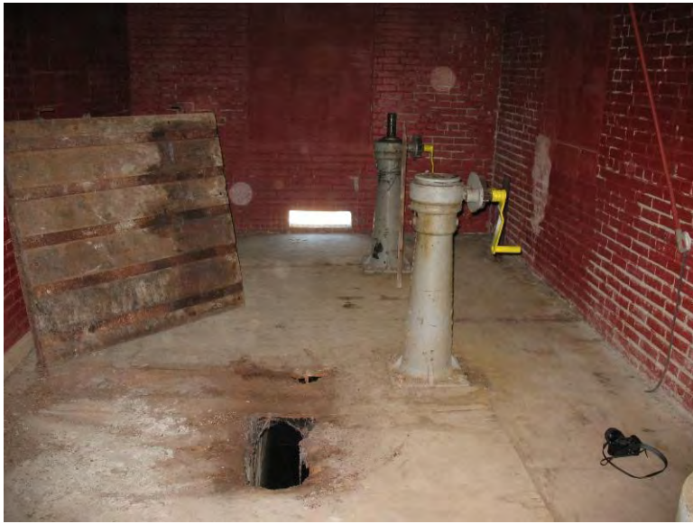
Photo 4. Turner Reservoir Dam. Low level outlet gatehouse with two floor gate operators.
