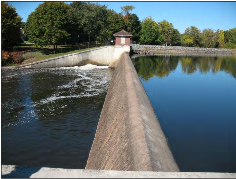
Photo 1. Turner Reservoir Dam. Spillway, outlet works, right retaining wall, and right dike from left embankment.
