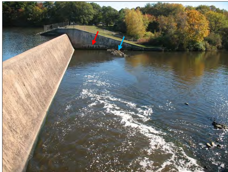
Photo 2. Turner Reservoir Dam. Spillway, left retaining wall, and left embankment from right river bank. Note horizontal crack in left retaining wall (red arrow), stone pile in tailwater (blue arrow), and vegetation at left embankment toe.
