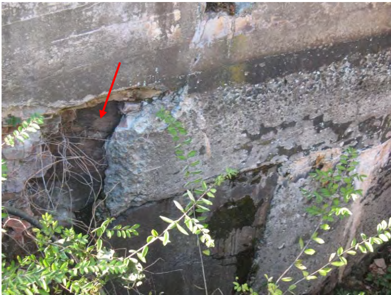
Photo 14. Hunt's Mill Dam. Concrete deterioration of riverside headrace open flume wall. Note stone masonry exposed due to missing concrete cover (arrow).
